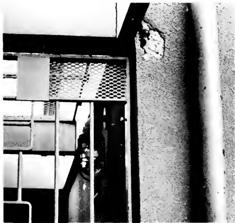
Photo 14. Fenton Avenue Elementary School. Slight damage to stucco where lunch-shelter roof joined multipurpose building.
